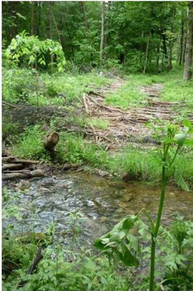
(a) Corduroy stream crossing at Timmouth Channel WMA reduces sediment erosion and dissipates stormwater runoff along road approaches to the creek.
