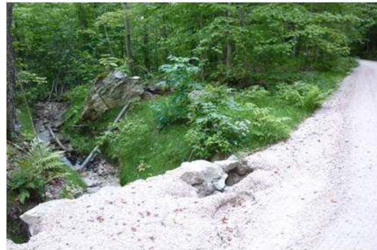
3. Erosion of road sediment from culvert header into tributary draining to Woodward Reservoir; site uphill from photo 1.
