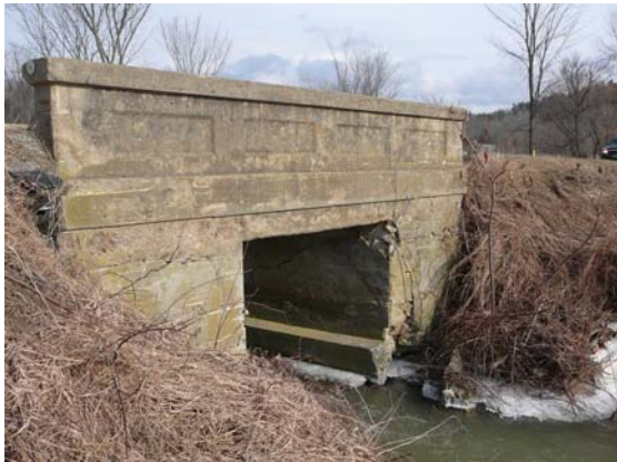
Figure 22. Concrete three-sided bridge, Spear Street crossing of unnamed tributary approximately 600 feet west of Quinlan Bridge; view of culvert outlet.
