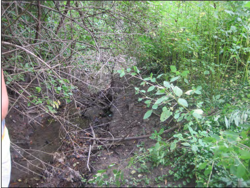
Figure 8. Eroding swale below outfall from Davis Avenue.
