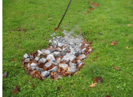
DRY WELL. This sand or gravel filled hole filters and infiltrates stormwater runoff. It is a great practice for properties with limited space.
